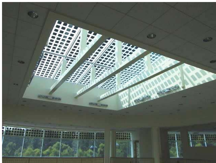
Fig. 4: BIPV skylight above entrance lobby
