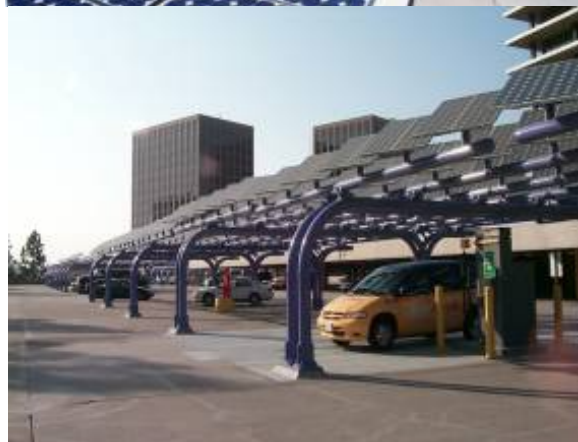
"Ra" - 150 kW system at LADWP headquarters: PV power, car shade, EV charging station
