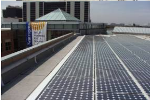
Neutrogena Corporation's 200 kW system Largest PV installation in Los Angeles
