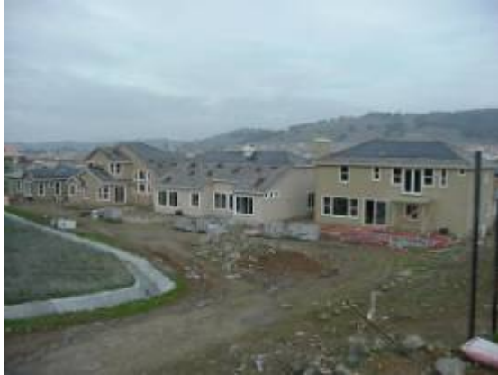
California building integrated residential roofing – 3 kW systems
