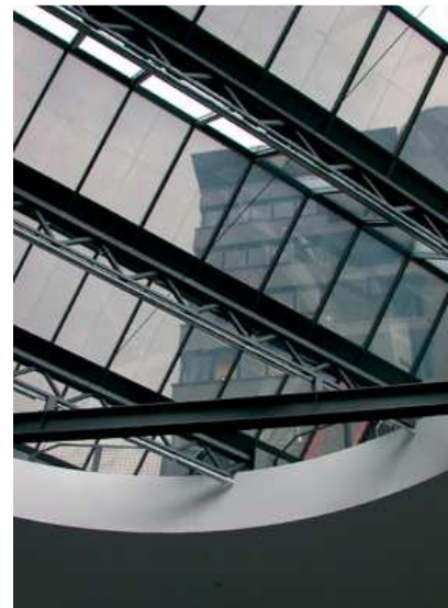
Illustration 4: PV-shed-roof: Photovoltaic shading (90%) with 10 % light entry by semitransparent amorphous PV-modules, which are integrated in the south orientated double-glazed shed-roof areas in the lounge of the local court in Kassel, Germany. [ISET]
