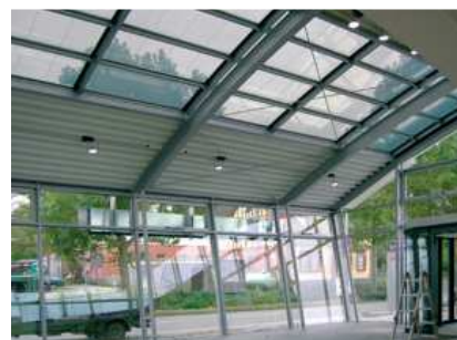
Illustration 6: Roof integrated skylight made of insulation glass components with semitransparent amorphous PV-cells in a showroom in Germany. [Glaswerke Arnold]
