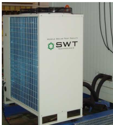
Fig. 2: Chiller connected to the container of the test facility
