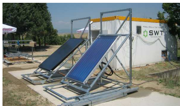
Fig. 7: Mobile, stand-alone test facility at Skopje, Republic of Macedonia
